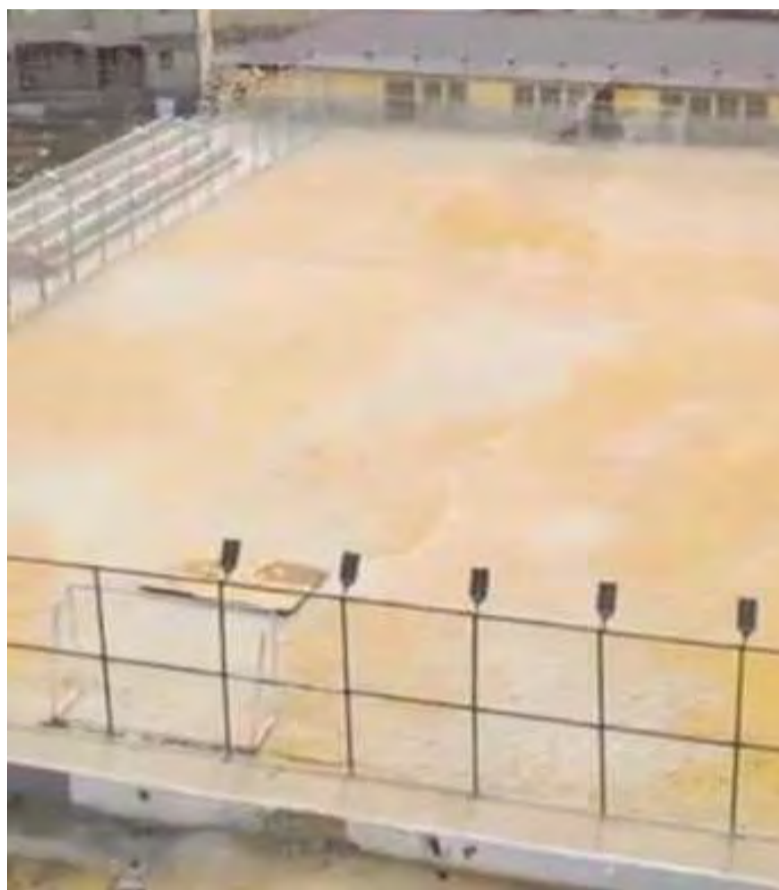
The ongoing construction of the Agboyi Town Elevated Football Pitch and Recreational Centre
